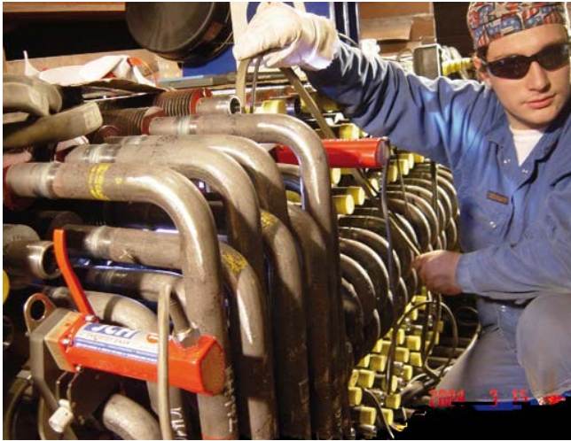
Fig. 2: For reliable connections between tubes, elbows and return bends in a tube bundle heat exchanger, orbital TIG welding is applied
