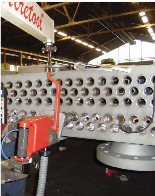
Fig. 15: TIG welding head with wire feeding device positions to weld a flush tube at the rear wall of a header box
